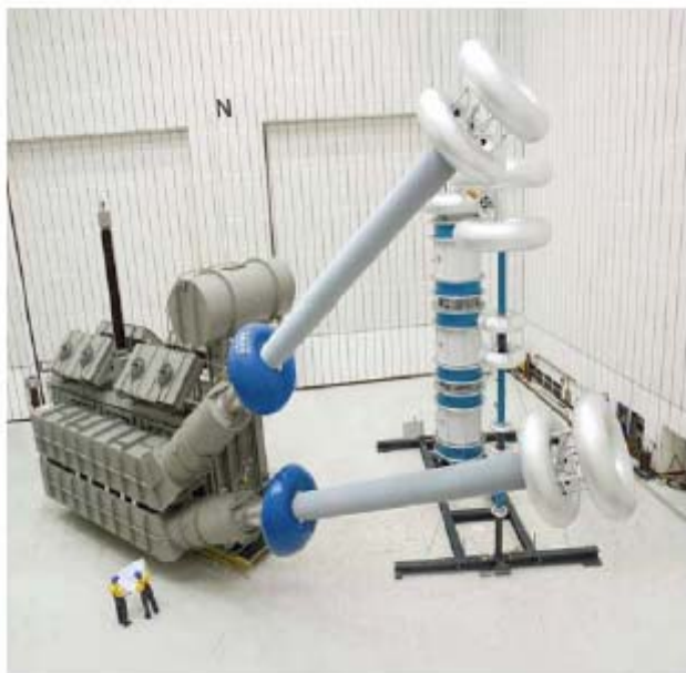
Figure 8: Converter Transformer for Yunnan-Guangdong Project in test field
